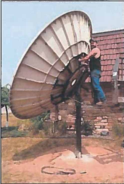
Ryan Halsey of Halsey Fabrications installed the dish necessary to broadcast Packers and Brewers games. Below: Another studio set-up is finished in Eagle River, ready for project completion to move WNWx Mix 96FM.
